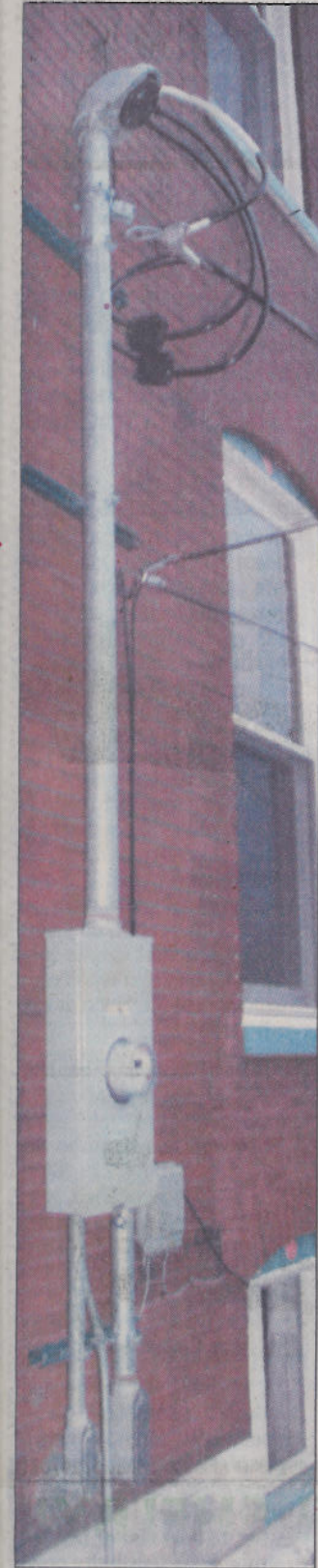
Electrical renovations included a new meter base and weatherhead on the home's exterior.
