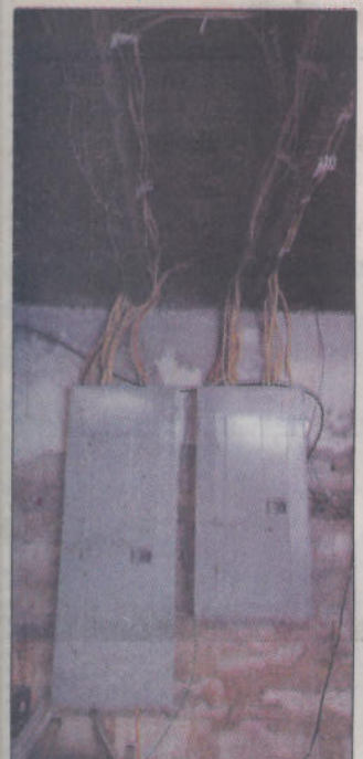
Circuit-breaker panel has a 320-amp electrical-current capacity.
