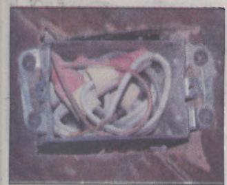
Floor outlets are commonly installed in historic homes that have solid-brick walls.
