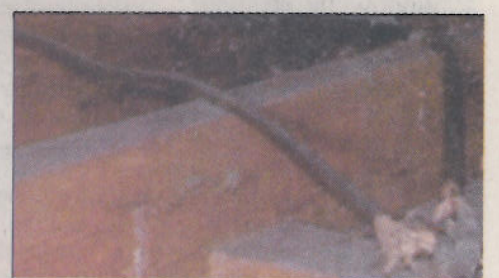
Old cloth-covered Romex wires.
